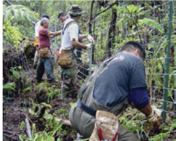
Fence being constructed to exclude feral pigs. Photo: Hawai'i Association of Watershed Partnerships.
